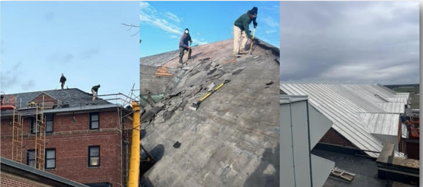
The before, during, and after of a new roof at Monastery Immaculate Conception in Ferdinand. The previous one kept the rain out for 80 years. Hopefully the new one will do the same.
